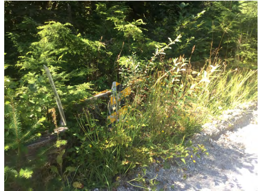
Right Approach Downstream Fender Partially Overturned
