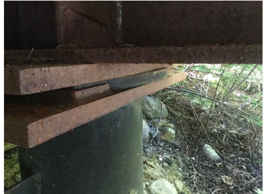
Typical Bulging of Bearings
