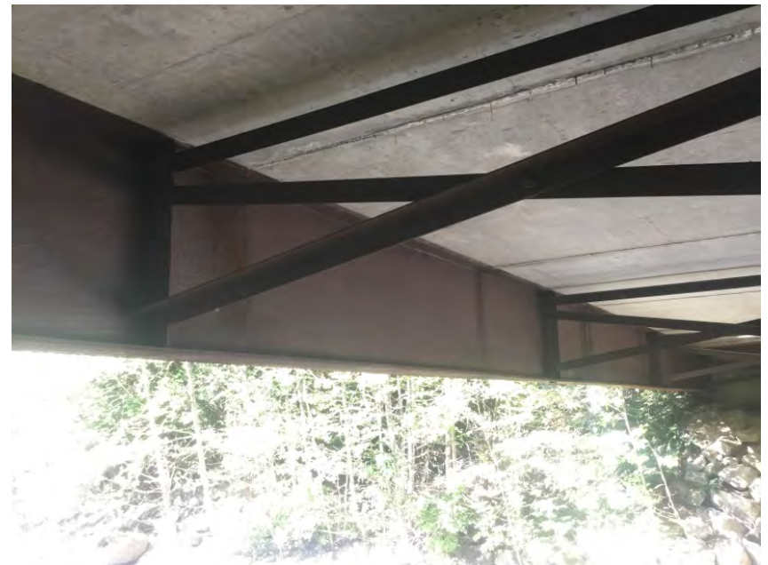
Girder Condition Noted Corrosion at Deck Panel Joints
