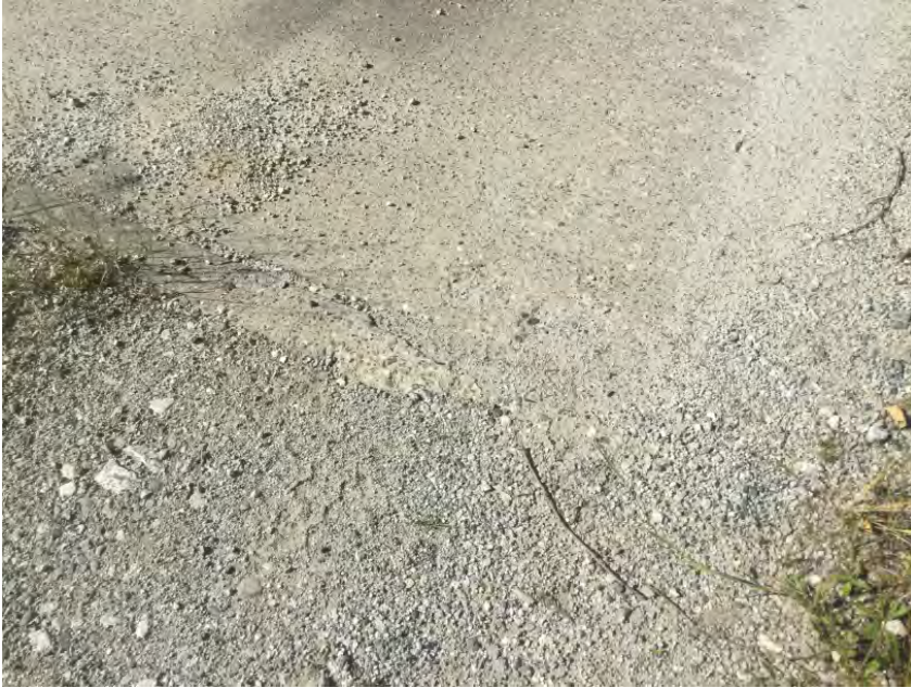
Typical Damage to Ballast Wall
